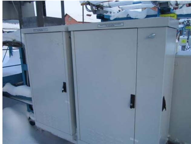
Figure 38. Main and BackUp PID cabinets installed at the 110 kV AIS [62].
